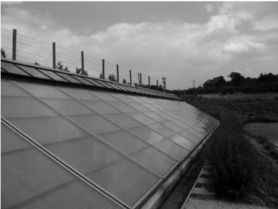
Solar Array, RES Group Head Office – Beaufort Court, Hertfordshire, England Hybrid thermal/photovoltaic solar energy panels. The system produces electrical energy and hot water [RES]
