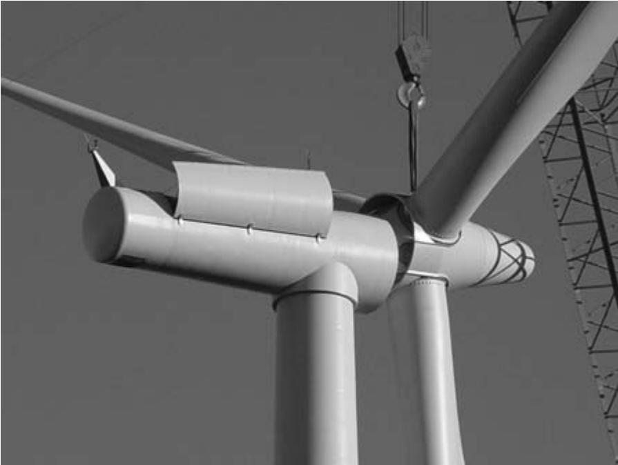
Nine Canyon Wind Farm, Tri-Cities, Washington USA (100 MW) Attaching the blade assembly of a 1.3 MW, active stall regulated, fixed speed induction generator wind turbine [RES]
