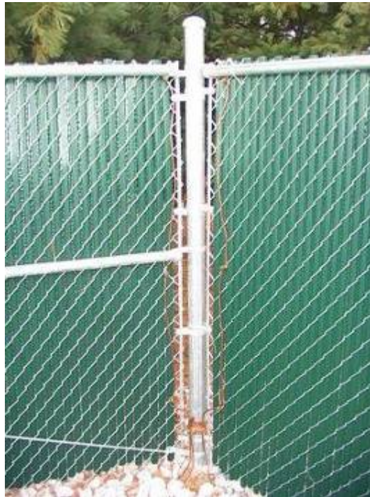
Figure 6-6 Example of Grounding Mat Tied to Fence Corner
