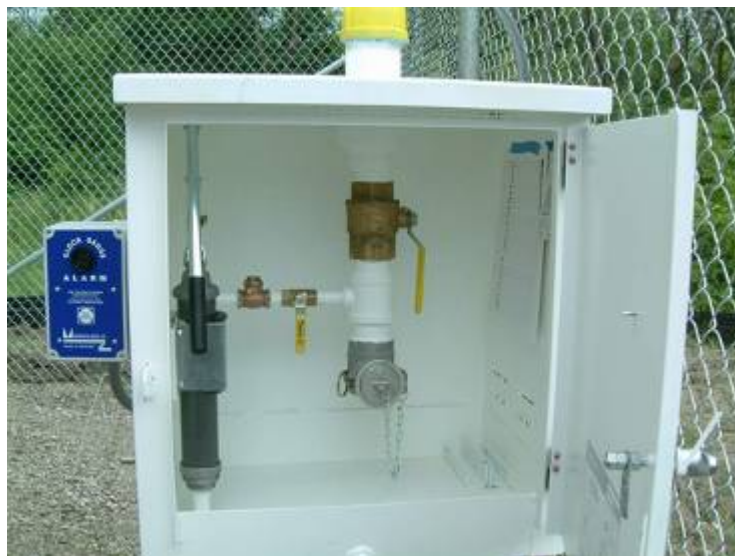
Figure 5-11 External Diesel Fill Box
