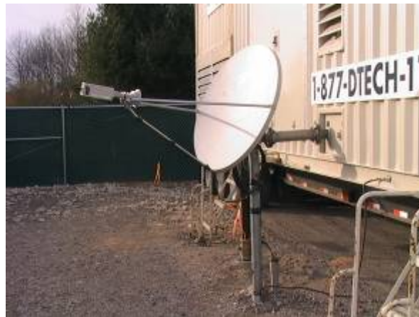
Figure 6-10 Example of Satellite Technology Being Used for Communications Path
