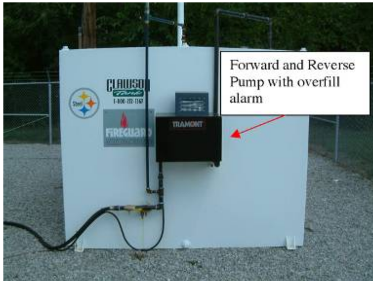
Figure 5-10 External 6000 Gallon Double Wall Fireguard Tank
