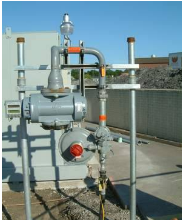
Figure 6-5 Example of a Natural Gas Meter for a 1 MW Generator
