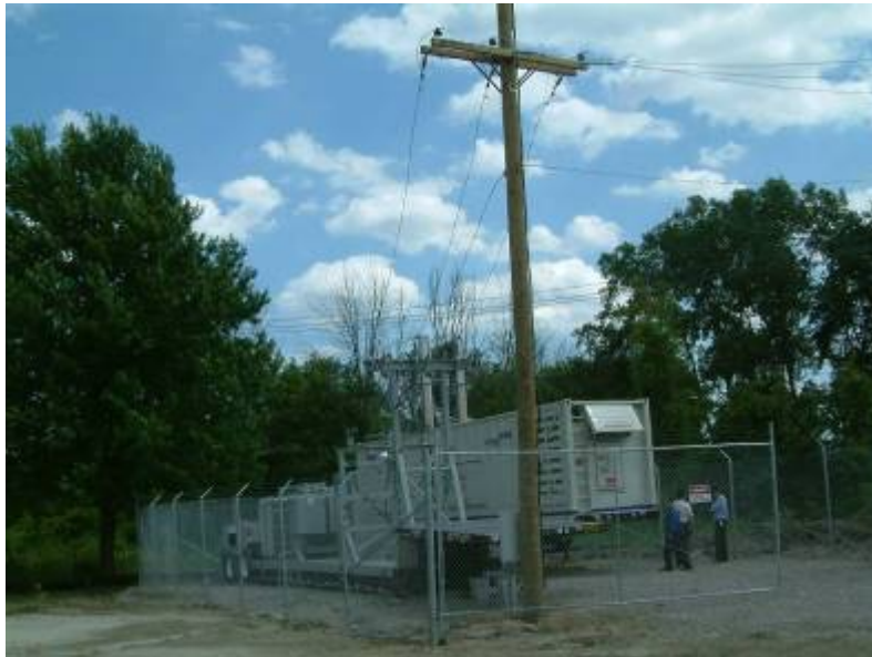
Figure 8-5 Wayne Emergency Installation
