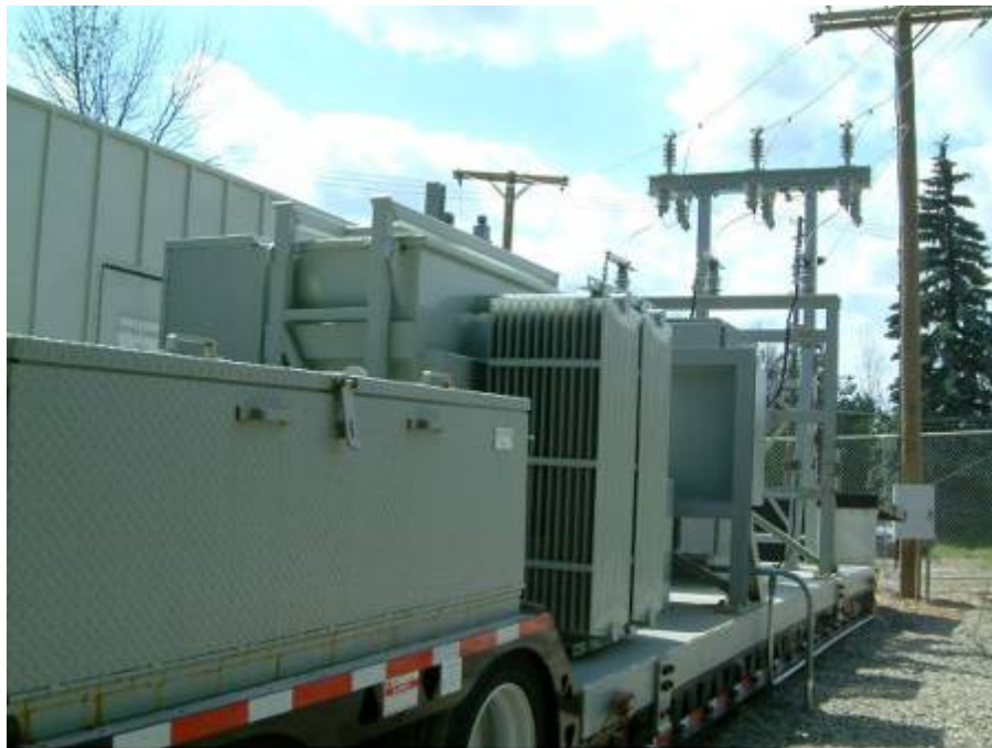
Figure 4-13 Interconnection Trailer for 4.8 kV and 13.2 kV Distribution Support
