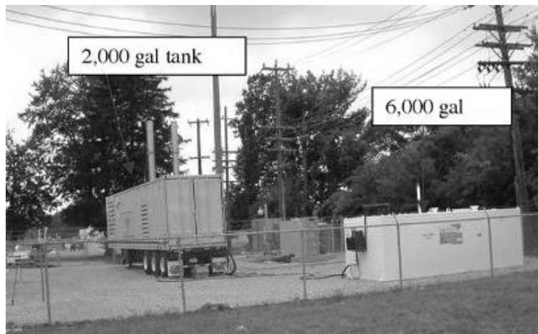
Figure 5-6 Internal and External Fuel Tanks
