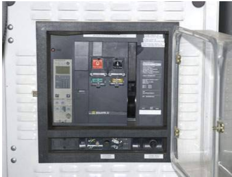
Figure 4-4 Square D Rack-out Breaker
