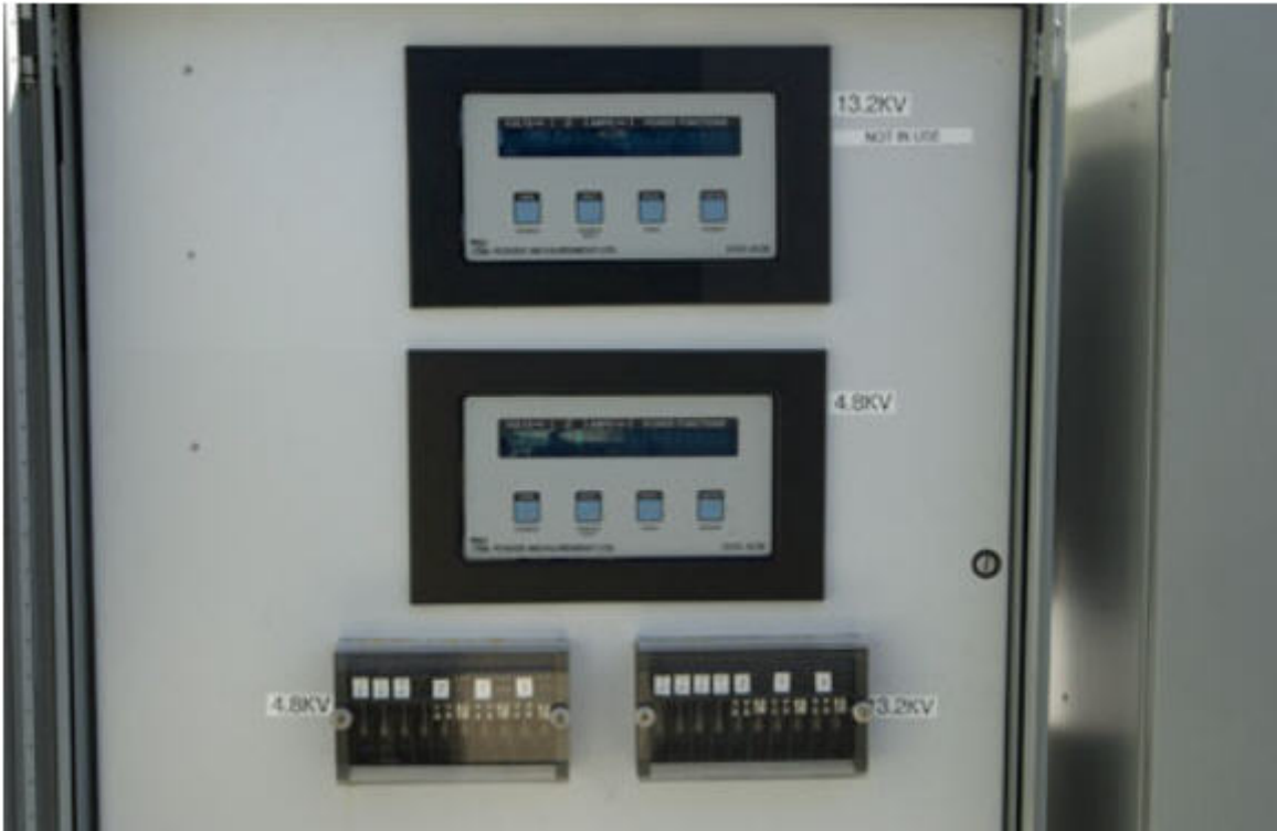
Figure 4-11 Skid: Metering Voltage Selection
