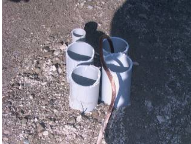
Figure 6-2 Underground Conduit for Connections Between Generator and Skid
