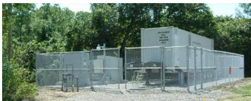
Figure 8-4 Grosse Ile 1 MW Natural Gas Generator to Defer T&D Expansion
