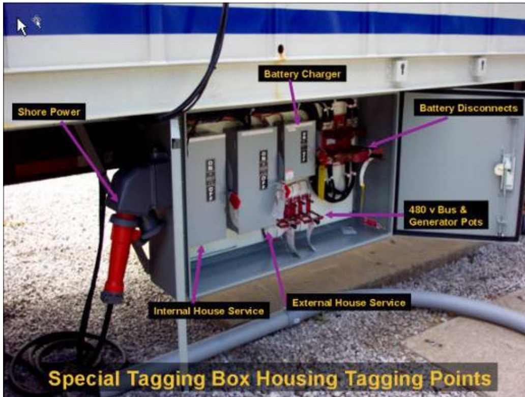
Figure 4-5 Tagging Point Box: Shore Power Connection and Visible Breaks
