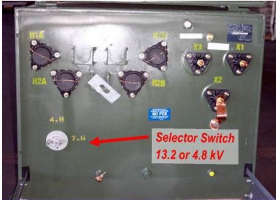
Figure 4-8 Skid: Dual Voltage House Service Transformer
