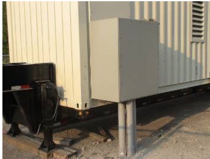
Figure 6-9 Example of Standing Doghouse for Interconnection Cables
