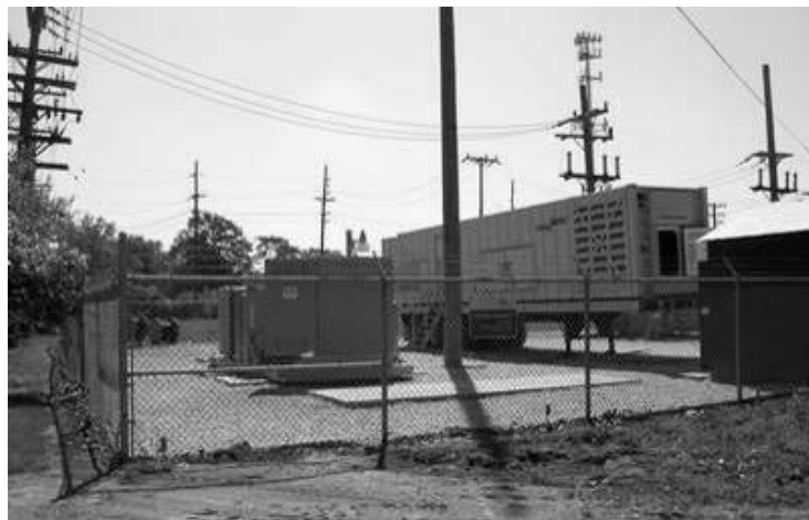
Figure 5-1 Example of DER Inside of a Substation
