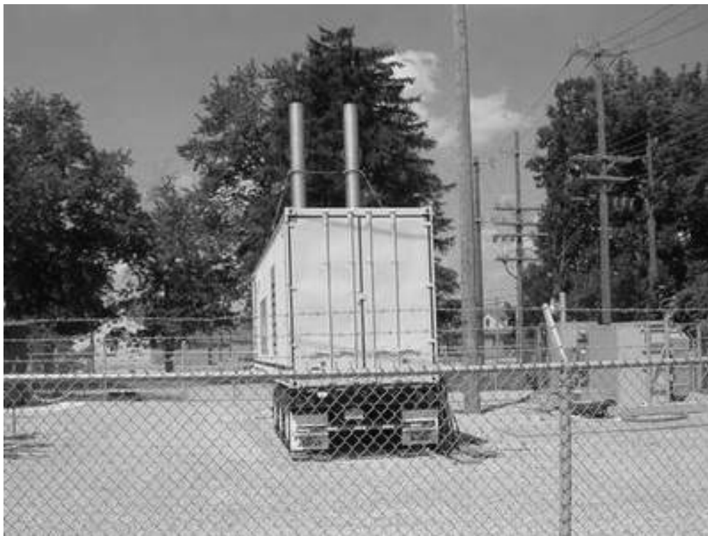
Figure 5-5 Example of a Generator With Stack Extensions
