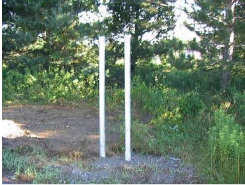
Figure 6-4 Example of Metal Support Posts for Natural Gas Meter
