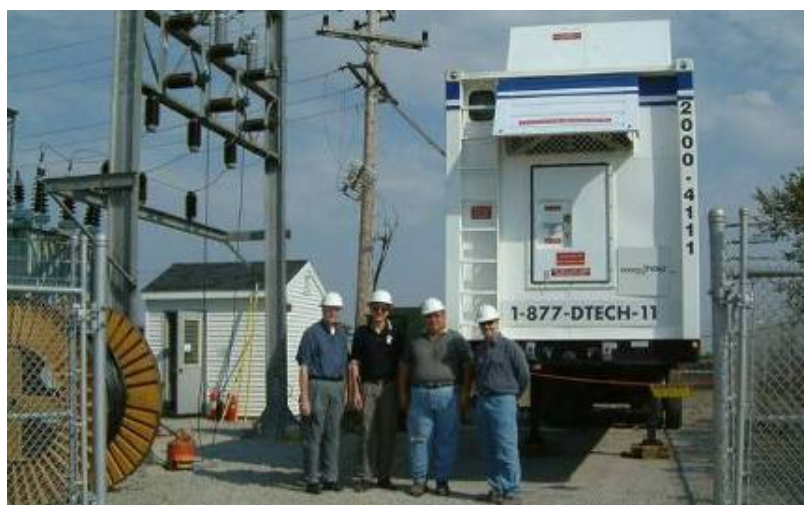
Figure 8-3 Quail Substation: 2 MW Diesel Installation to Support Maintenance Shutdown
