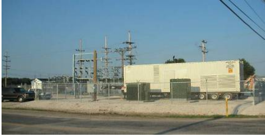
Figure 8-2 Adair Temporary Installation
