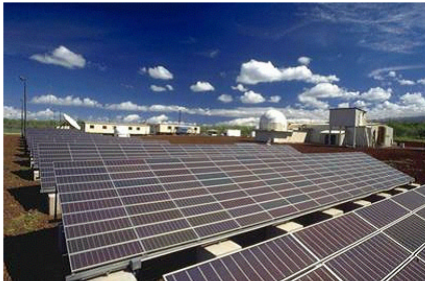
Figure 6-1 PVUSA 20-kW Facility in Kihei, Maui
