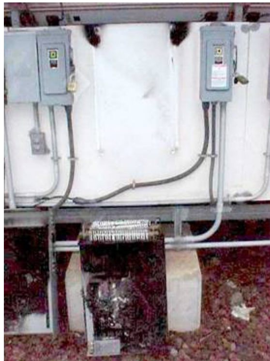
Figure 6-4 Photograph of the Board to Which the Damaged Omnicion Inverter was Mounted (Note the two Burn Marks at the Top of the Board)
