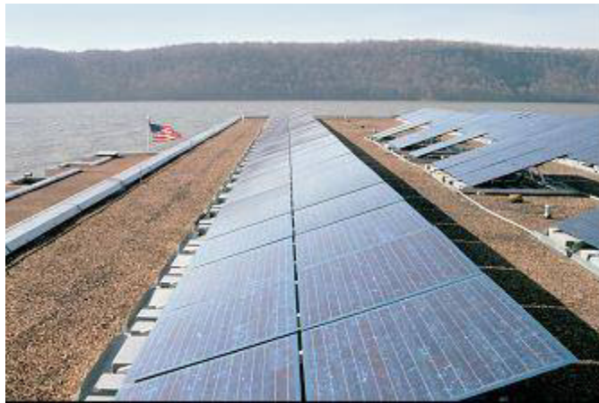
Figure 3-7 Roof Mounted PV Installation at the Yonkers Wastewater Treatment Facility
