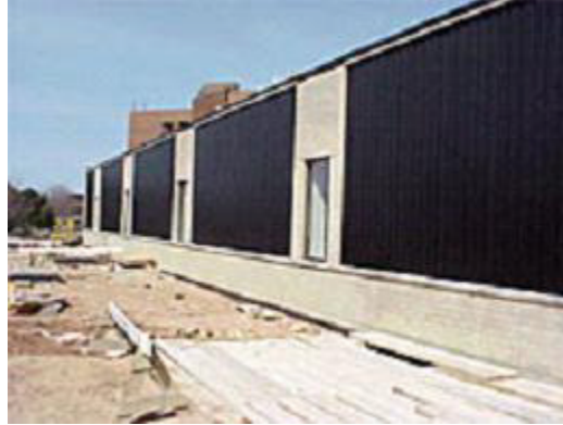
Figure 4-6 The South Facing Wall of Mary Ann Cofrin Hall Incorporates Solar Wall Heating Technology
