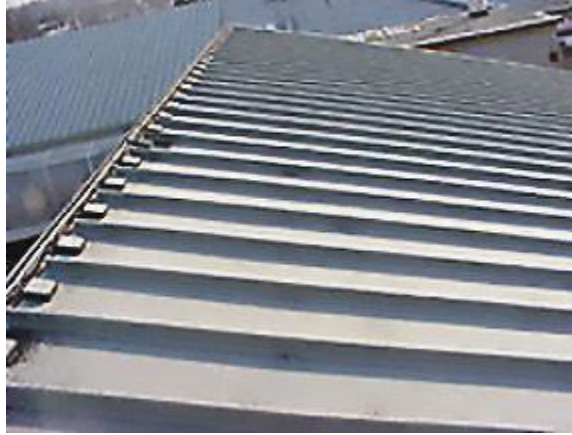
Figure 4-3 Completed Installation of PV Standing Seam Metal Roof on Mary Ann Cofrin Hall
