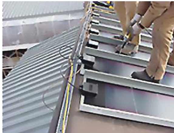
Figure 4-2 Installation of PV Standing Seam Metal Roof on Mary Ann Cofrin Hall
