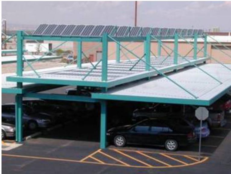
Figure 5-1 Parking Structure Photovoltaic System at the PNM Facility in Albuquerque, New Mexico
