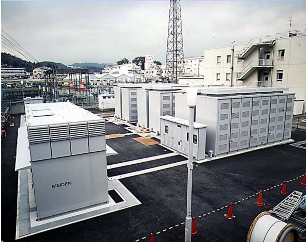
Figure 2-2 6 MW / 48 MWh NAS System at TEPCO Ohio Substation
