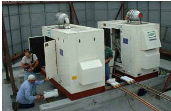
Figure 3-3 Two Hess Internal Combustion Engine (ICE) gensets integrated into a Turnkey Cogeneration Package by RealEnergy
