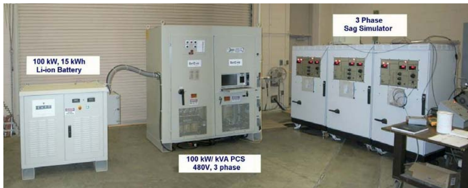
Figure 3-8 Li-ion UPS Systems - 100kW, 30s
