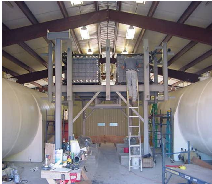
Figure 3-9 Vanadium Redox flow battery 250 kW 8 Hrs installed at PacifiCorp site at Castle Valley, Utah
