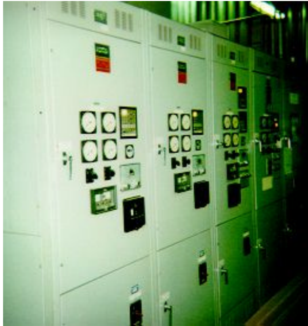
Figure 3-9 Generator Control Panels, External
