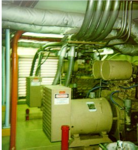
Figure 3-7 Two 450 kW Cummins Diesel Generators (Gen 1 and 2)
