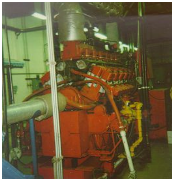
Figure 3-8 800 kW Waukesha Generator (Gen 3)
