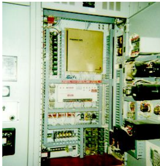
Figure 3-10 Generator Control Panels, Internal, Showing ENCORGPC unit (upper right)
