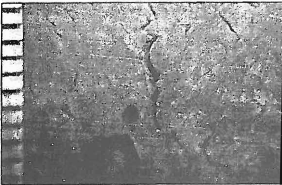
Figure 12 Cracked lead sheath of a PILC cable.
