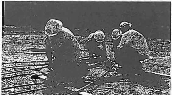
Crew prepares for pulling wire by installing grips that will attach the wire to the running board lying on the ground. The running board is pulled through the blocks laying the six conductors in the proper wheel of the stringing block.
