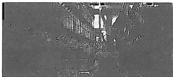
The 'world's most largest battery': Golden Valley, Alaska, Ni-Cd battery energy storage system. (Patrick Endres/Alaska&PhotoGraphics.com)
