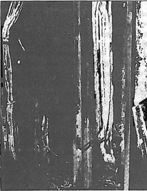
Figure 1 Burndown damage caused by arcing fault. View shows low-voltage cable compartments of secondary unit substation.
